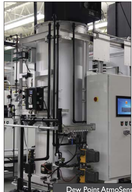
Dew Point AtmoSense™ on Endothermic Gas Generator
